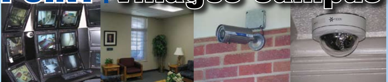
Video surveillance technology from Vicon includes infrared cameras (middle right) and impact-resistant mini-dome cameras (far right), which are monitored from a central command center (far left).
